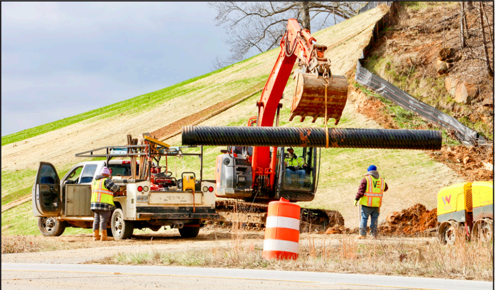
The Vertical Earth construction company is aiming to keep commuters happy as crews work to finish Phase II of GA 515 reconstruction as quickly as possible. Photo by Shawn Jarrard
