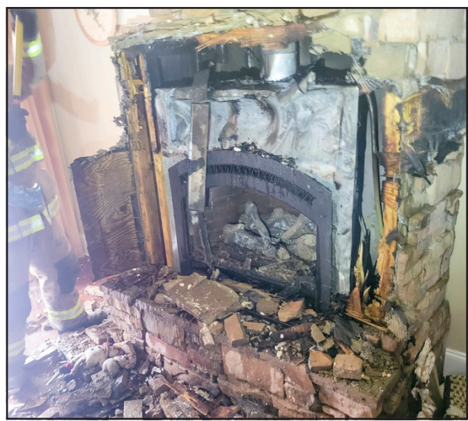
The Hawks Harbor fire started in the chimney chase of this fireplace, which had to be gutted to put out flames in the wall.
