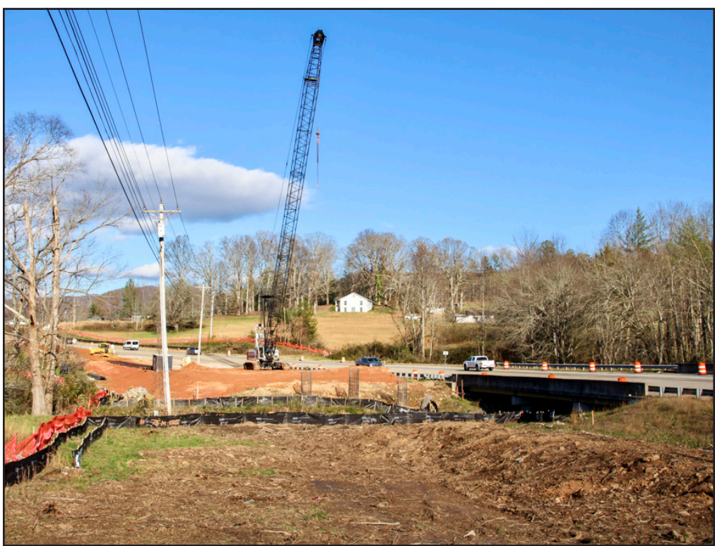
Construction of the new bridge over Brasstown Creek at the county line continues apace as part of the GA 515 project. Photo by Shawn Jarrard
